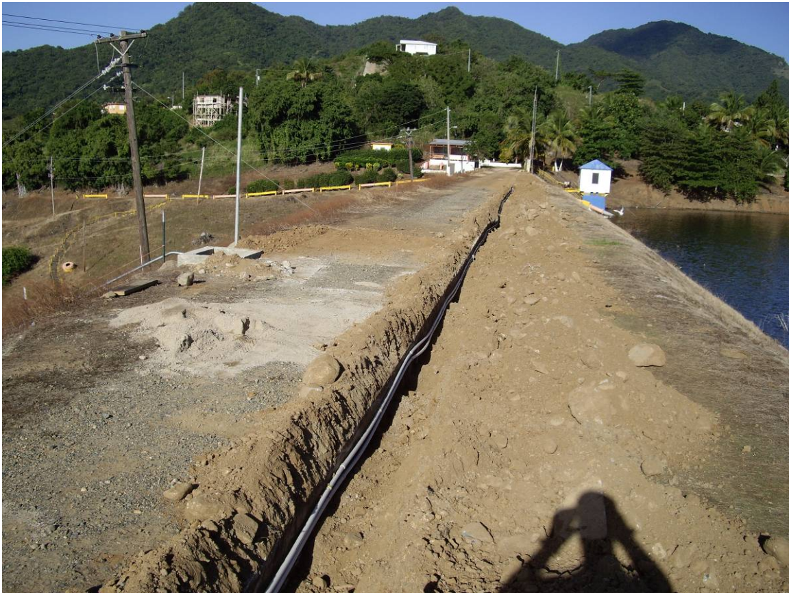
Figure 3-5. Picture of Underground Pipes
