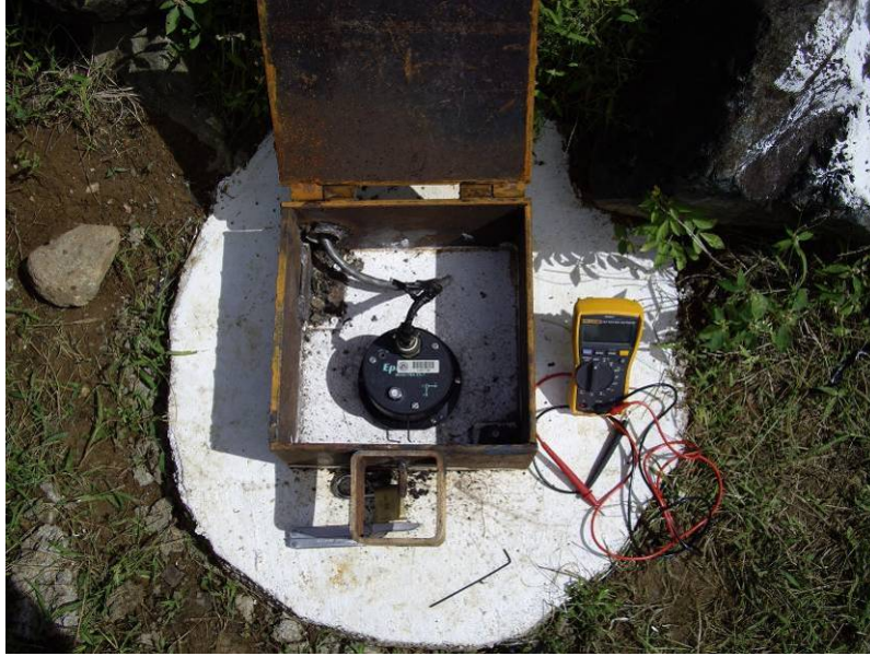
Figure 3-7. Triaxial Sensor at the Toe of the Dam
