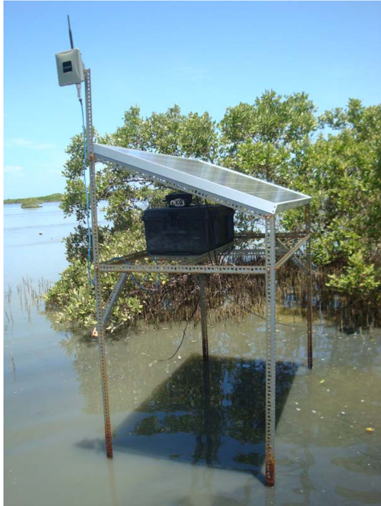
Figure 5–4: Testbed Installed in the Mangrove Area, Wireless Antenna, Solar Panel, and MSN Pelican Box are visible
