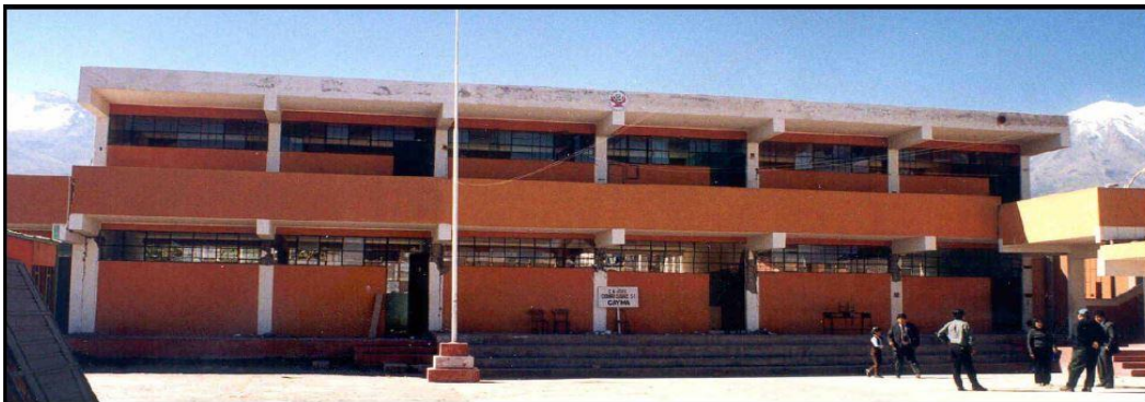
Figure 18. School building before 1997 damaged in the Atico earthquake, Peru, 2001.
