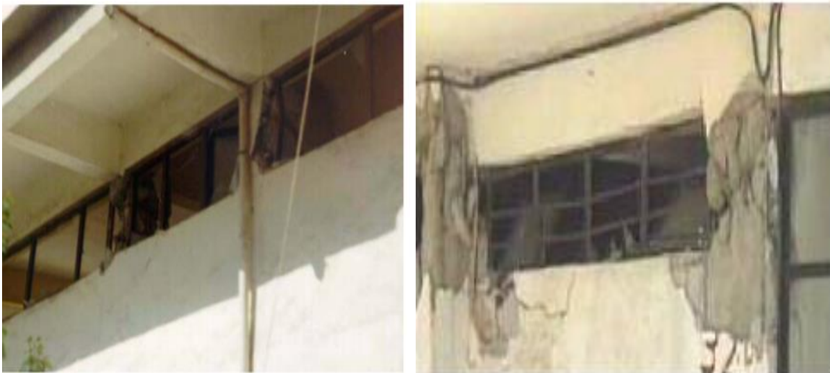
Figure 10. Damages due to the short column effect in the Izmit Earthquake, Turkey 1999.
