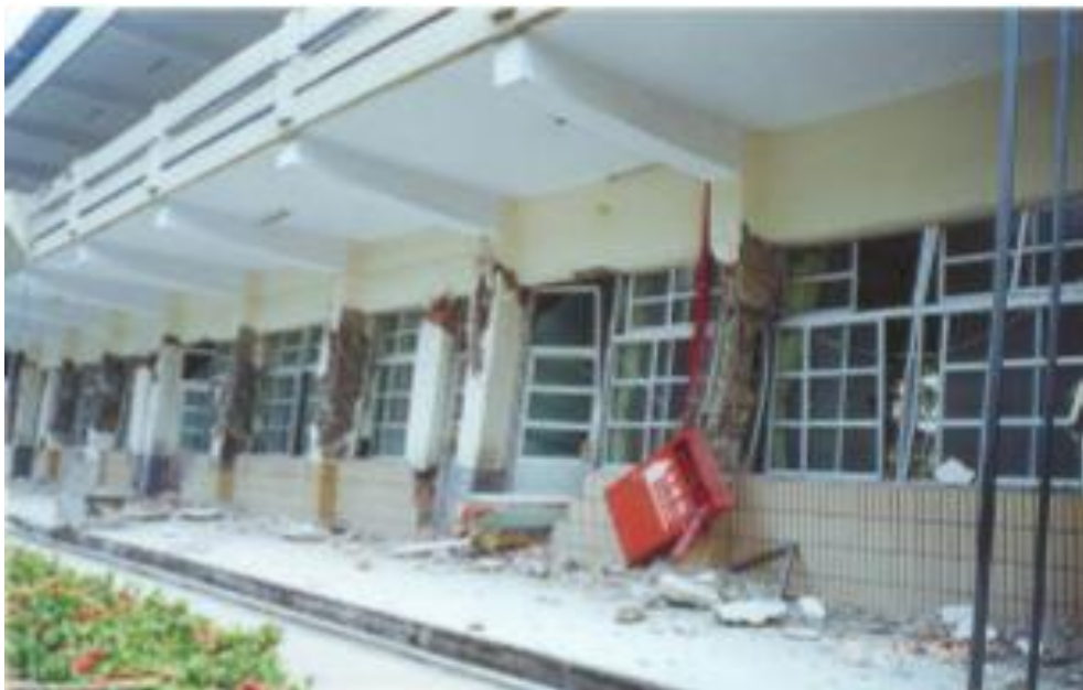
Figure 11. School damaged due to the short column effect.
