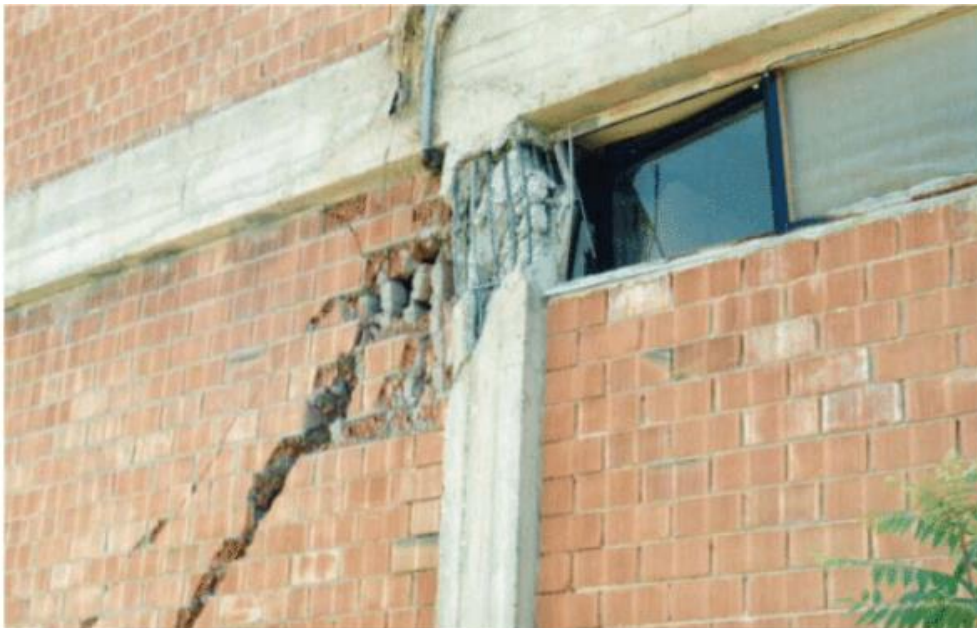
Figure 9. Short Column failure in the Adana Ceyhan earthquake, Turkey, 1998.
