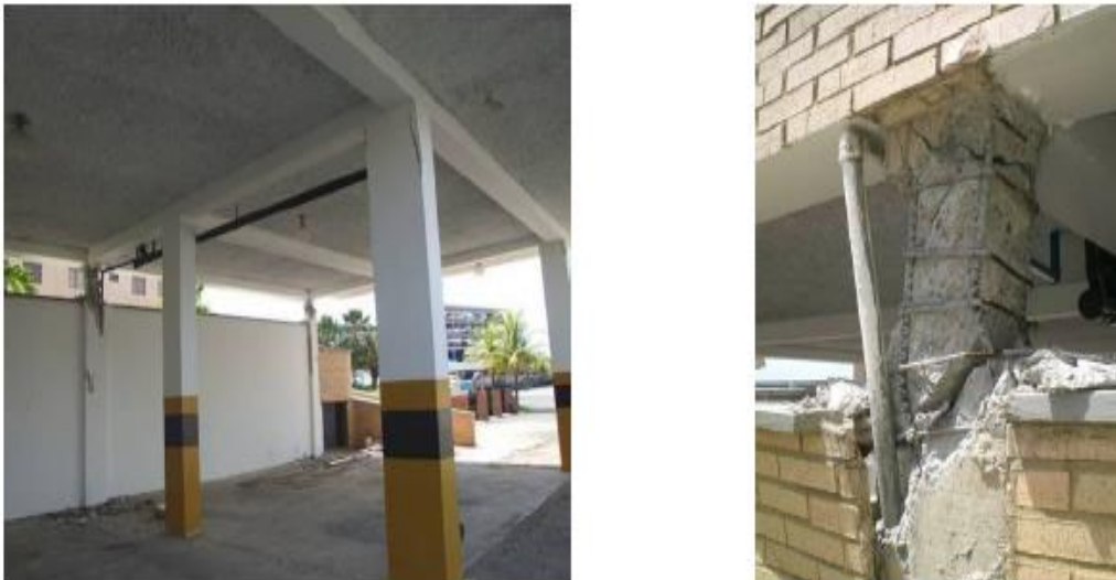
Figure 12. Short Column effect generated by reinforced concrete walls in a building in Tucacas, Venezuela during the September 2009 earthquake.
