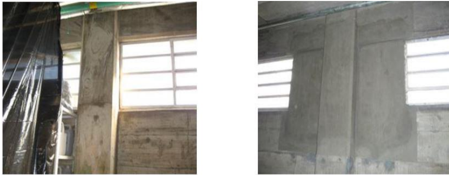
Figure 16. Incorporation of infill wall segments on both side of the short columns.
